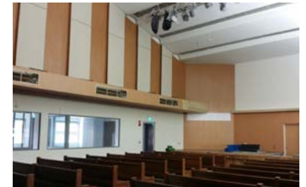
Worship Hall with re-varnished pews now in place. There are still some touch-up works to be done at the front stage area.
